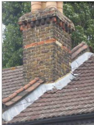
Photo - 3 Front chimney stack- worn pointing
