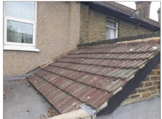
Photo - 5 Rear outrigger- fair order but a number of different flashings have been used around its perimeter and these can sometimes be difficult to bond
