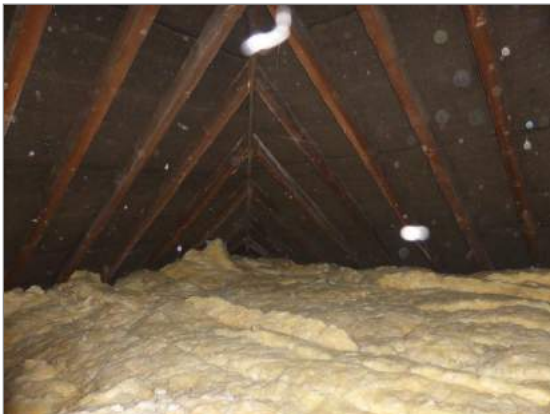
Photo - 8 Main roof frame- fair order
