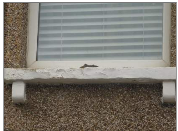
Photo - 7 Front window ledge- fine cracking and flaking paint
