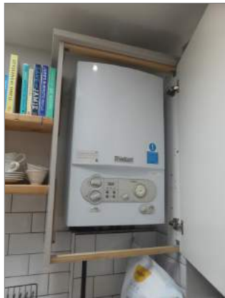
Photo - 17 Mid range combination boiler
