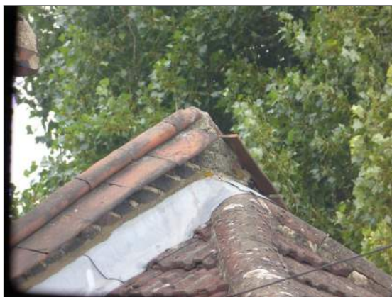
Photo - 6 Damage to parapet ridge copings
